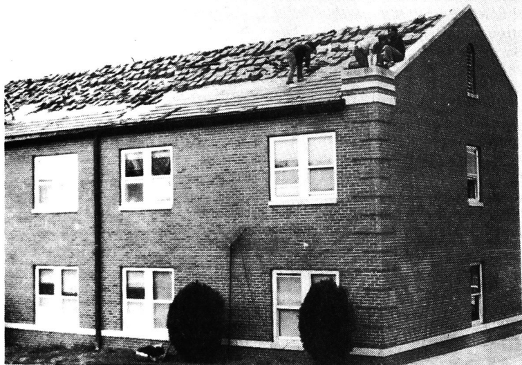
Neff Hall, the oldest men's dormitory on the campus of Southwestern State University, is in the process of being remodeled, according to Dr. Fred Janzen, Dean of Student Personnel Services.
